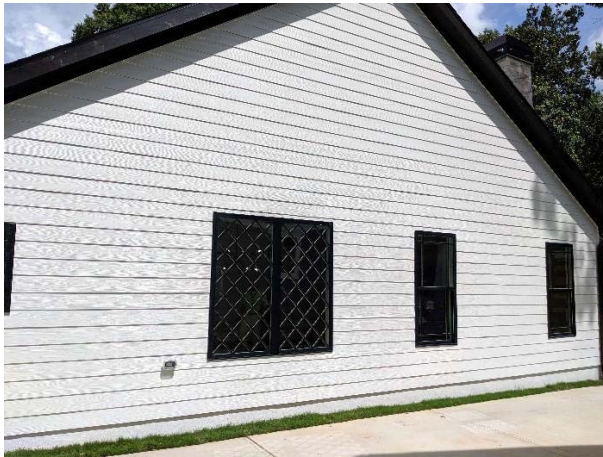
Left elevation, showing unapproved window, compared to plans.
